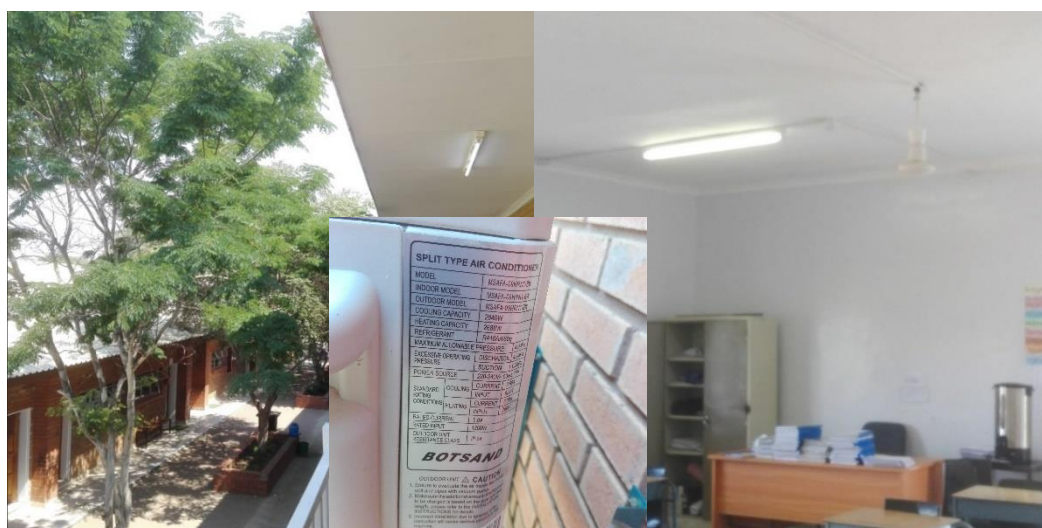
Figure 4: Observed energy waste and the energy data for the aircon used at Regent Hill School.
