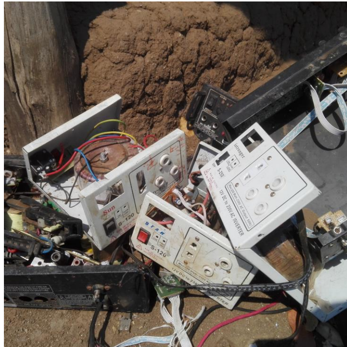
Figure 8: Damaged inverters used in a household in Majwanaadipitse.
